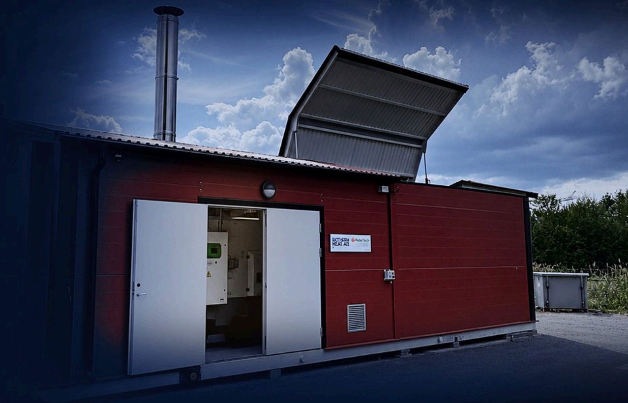
HEATING PLANT WITH BUILT-IN FUEL STORE, ROOF HATCH OPEN
