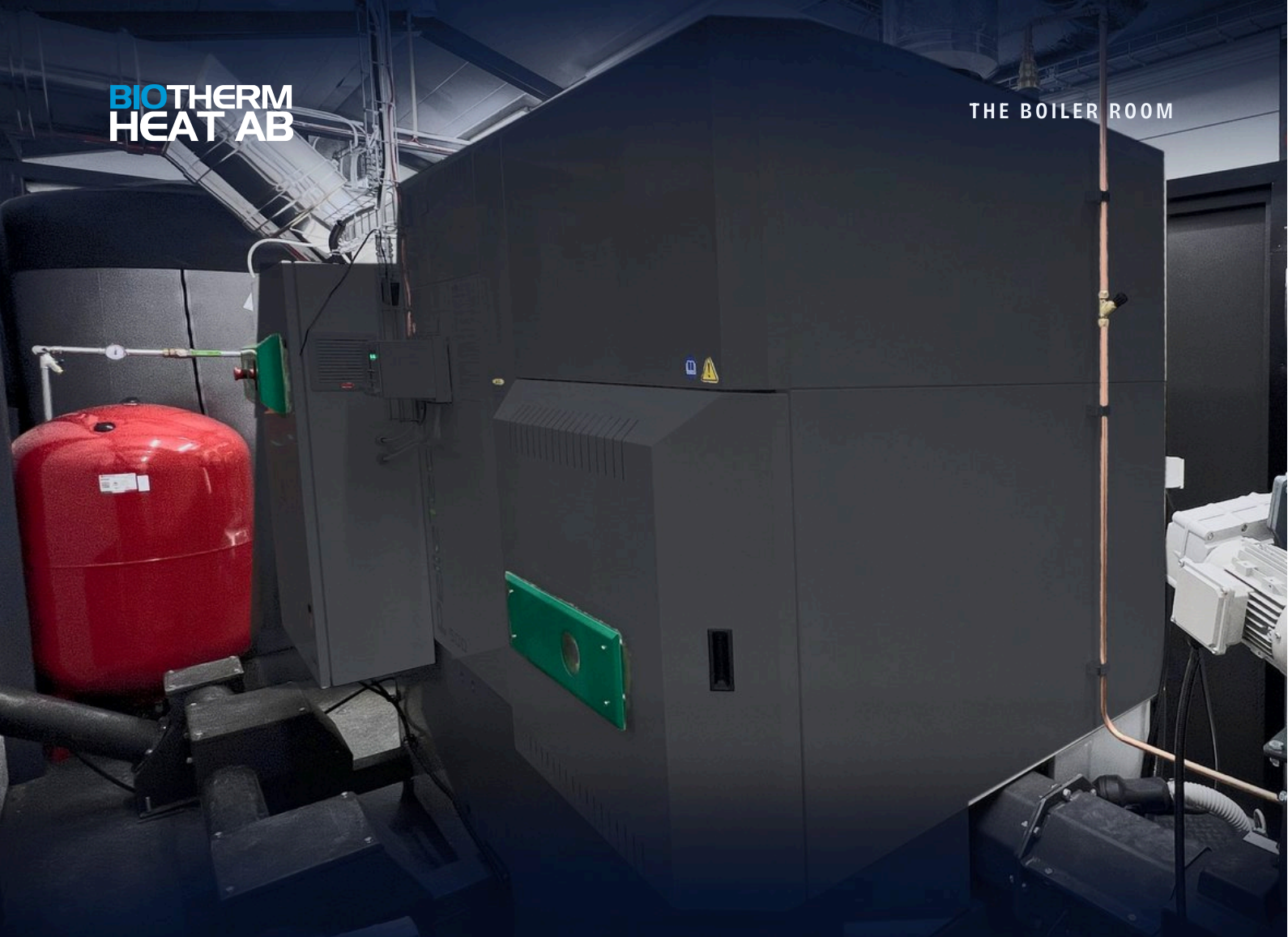
PELLETECH IDRO 500 IN A DELIVERED HEATING PLANT
